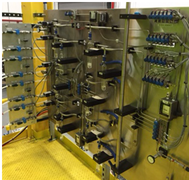
FIG. 2. Hall D gas panel.
